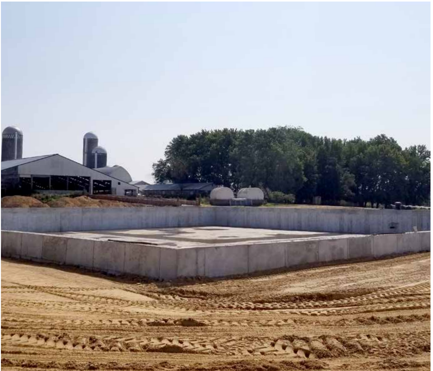
Vertical concrete waste storage facility with push off ramp. Courtesy of Chippewa County.
